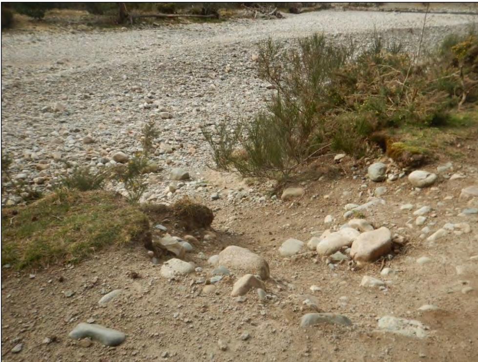
Plate 22 Partial breach of embankment at 36133,95261 (2022)
