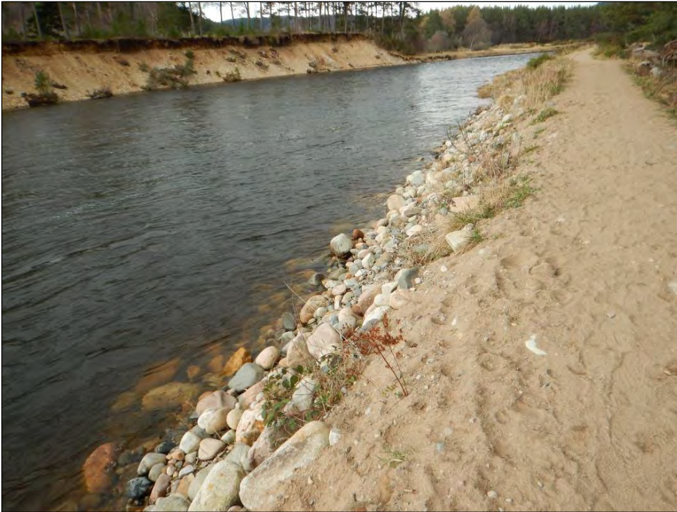
Plate 29 Unvegetated face of re-profiled embankment (2018)
