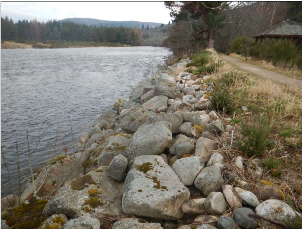
Plate 41 Exposed cobbles/boulders on river side of embankment at 14th Tee (2022)
