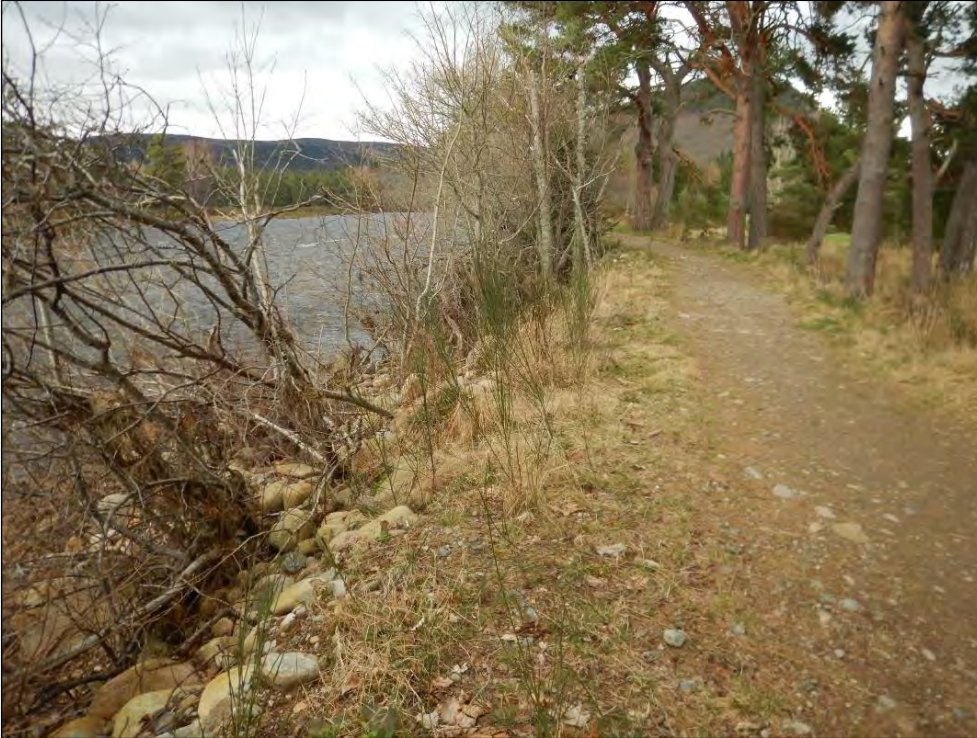
Plate 34 Embankment south of the 14th Tee showing exposed cobble (2018)
