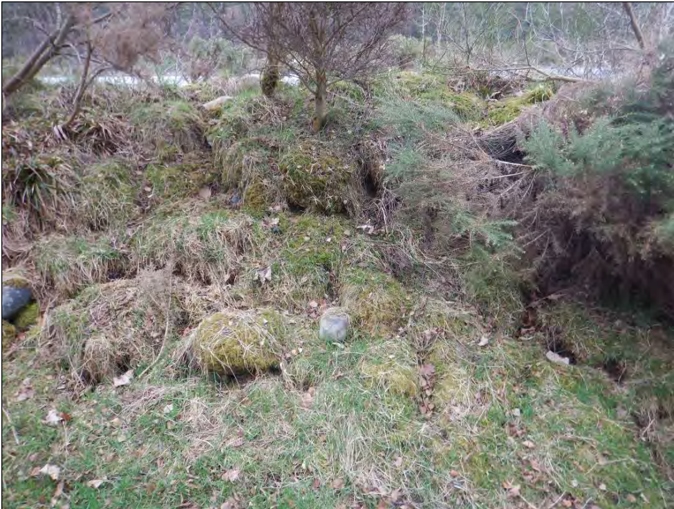
Plate 50 Holes in raised embankment (2018)
