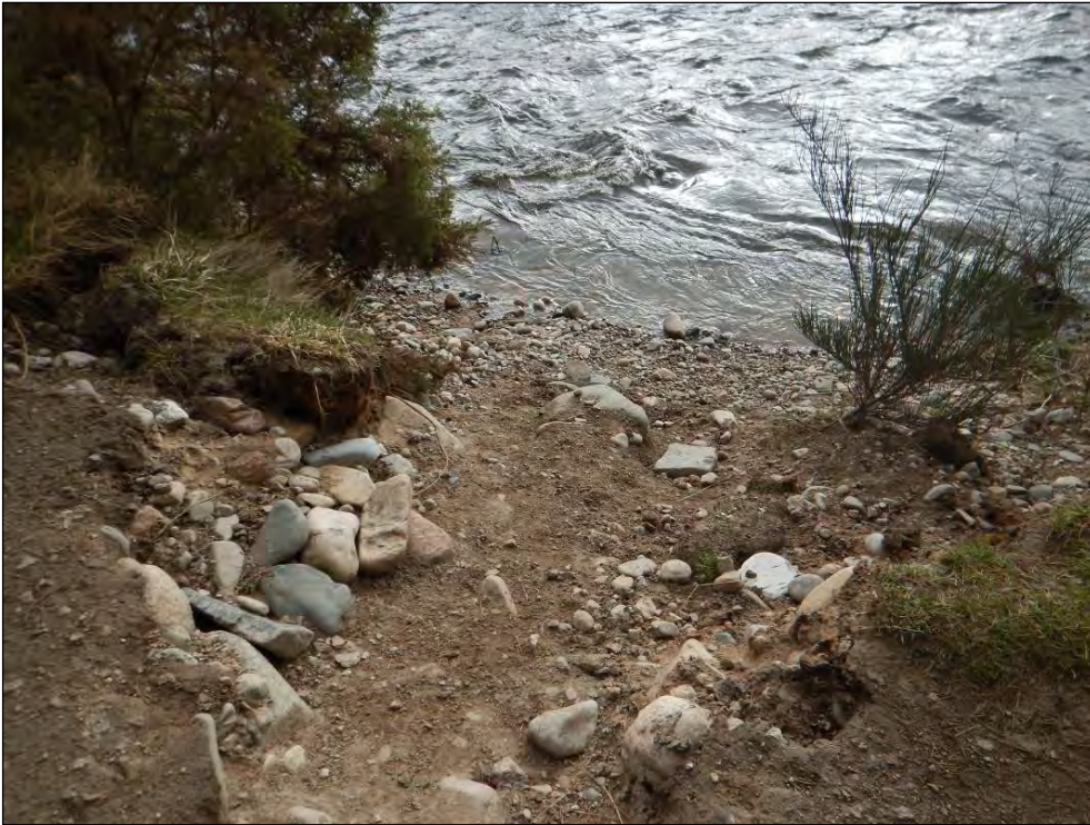
Plate 19 Partial breach of embankment at 36133,95261 (2018)
