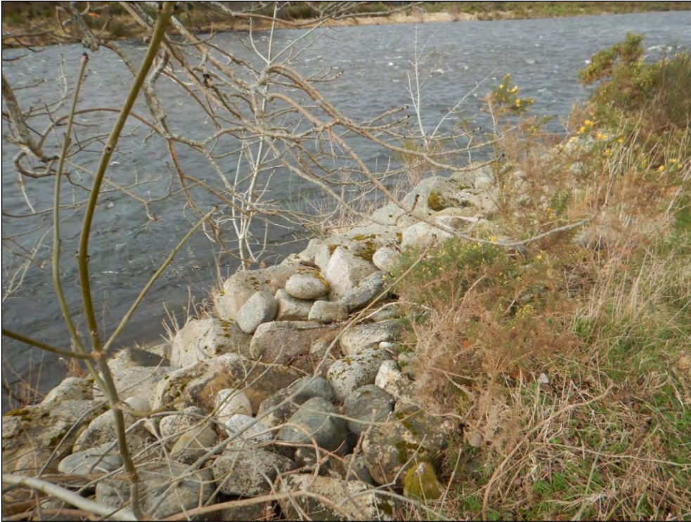
Plate 40 Exposed cobbles/boulders on river side of embankment at 14th Tee (2018)
